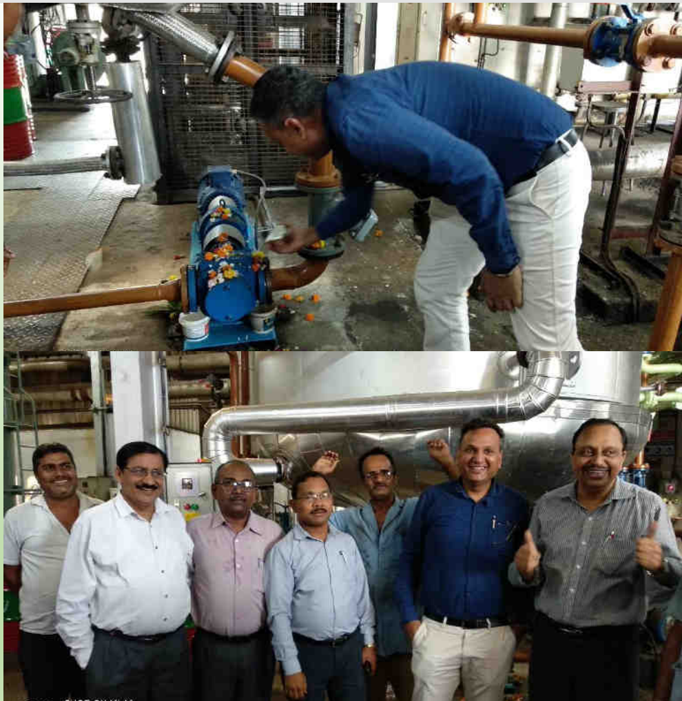
An Ester Blending Kettle of 12 MT capacity was installed at the Ester Plant in Greases & Lubricants, Kolkata and inaugurated in the month of April 2019.
