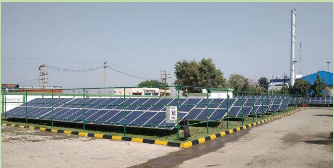
Solar power plant
